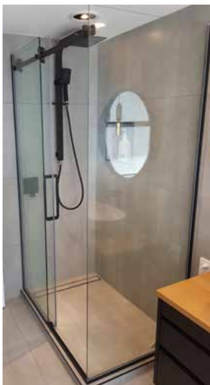
Pictured here - Black Premier Frameless Sliding Door 1200x800 onto small hob, tiled floor and walls.
